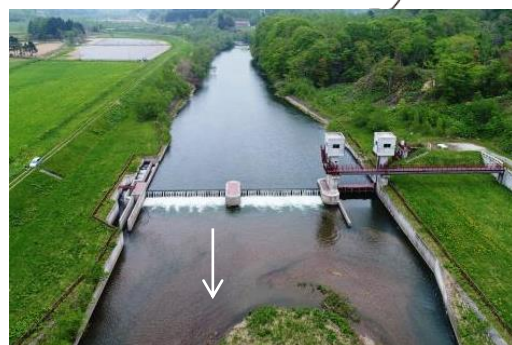
②中里頭首工(魚道)
