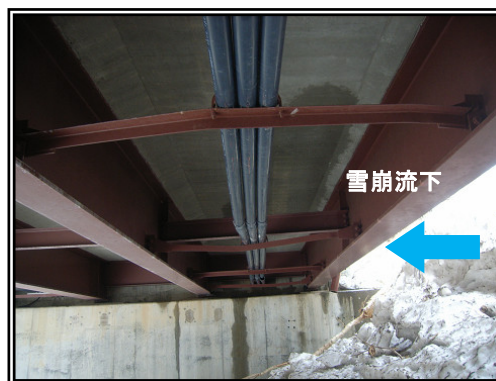
[山側主桁変形]
