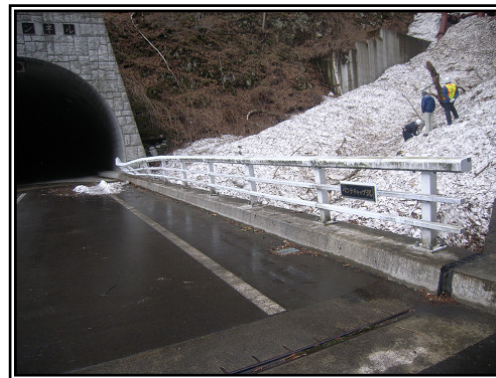
[山側防護柵変形]
