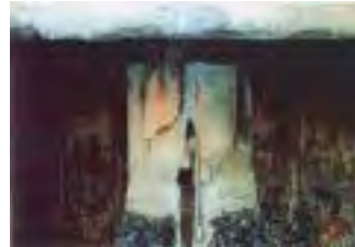
岸壁PC杭の亀裂
