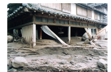
Damage Caused by a Rainfall-Induced Volcanic Mudflow (Mount Unzen-Fugen) (Courtesy of Shimabara City)
